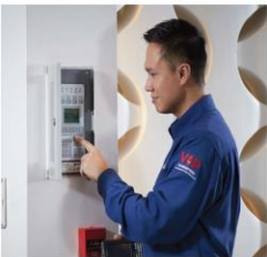
Fire Alarm and Monitoring
