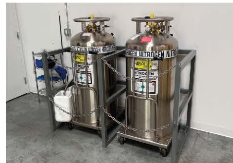
Gas Cylinder Storage
